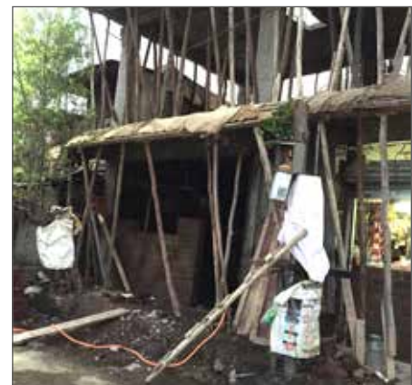
FIGURE 23: ADDITION OF A FLOOR IN A NOTIFIED SLUM IN PUNE
